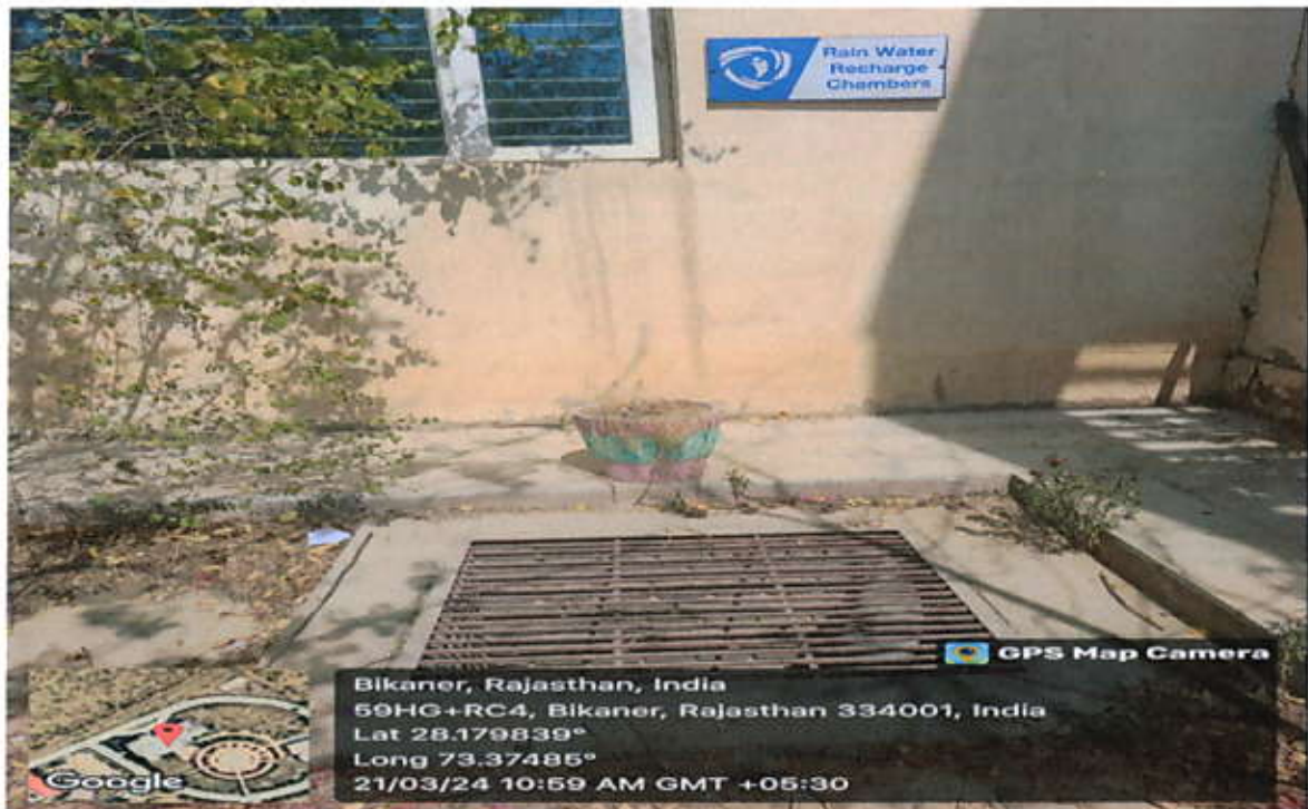
Rain Water Recharge Chambers
